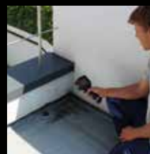
Discover leaks in roofs
